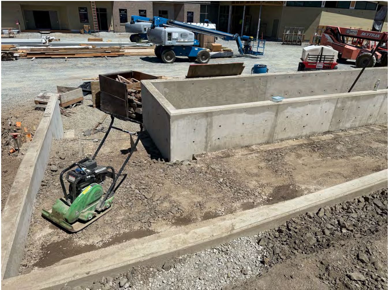
Fig. 3) Preparation of ramps and walkways at the front of the building/parking lot.
